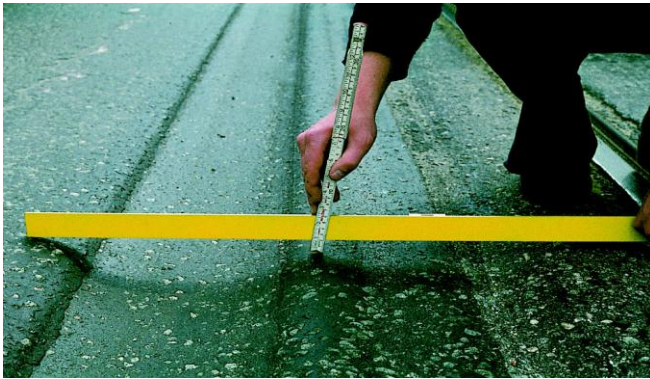
Rutting caused mainly by studded tire wear
