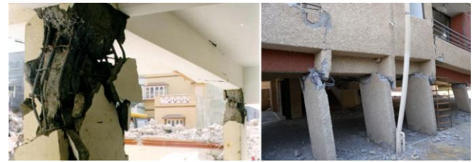
Fig -5: Damages in columns during earthquake
