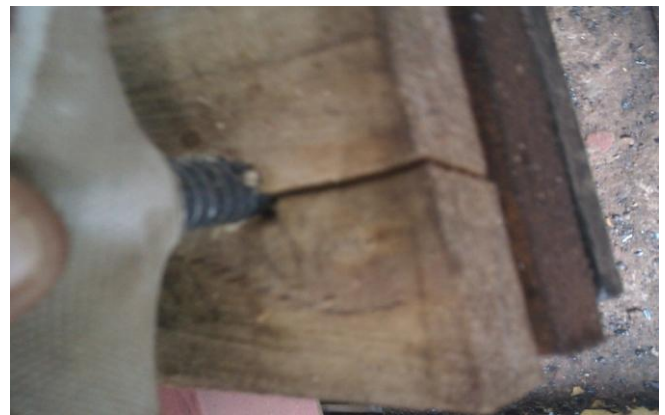
Fig- 1.4: Crack Prorogated near Discontinuity of Wood Plank
