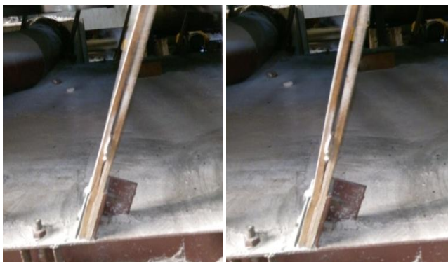
Fig-1.3: Wooden Plank-Before and After Failure
