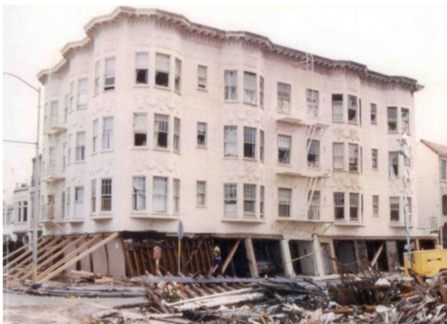
Figure 2 – Failure of multi storey building due to soft storey at parking level.
