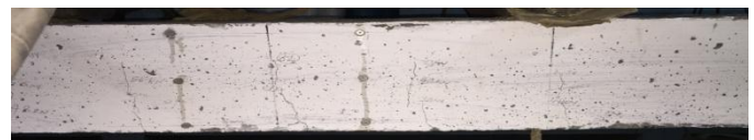
Fig 5: Cracking pattern of beam CB
