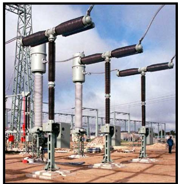
Fig -1: Switchgear in working condition
