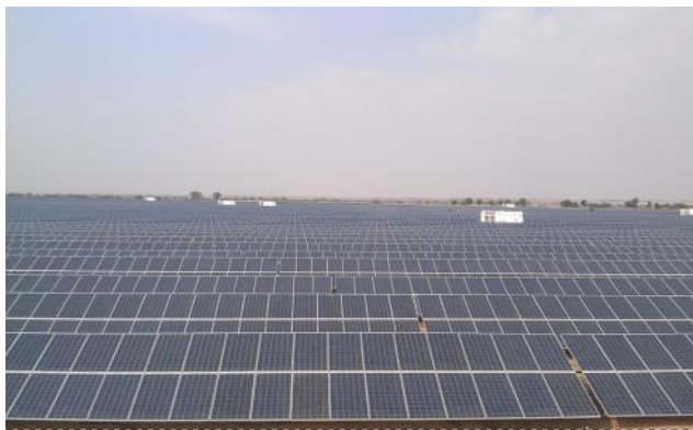
Fig-2: 10 MW Solar Power Plant, Kolayat, Rajasthan
