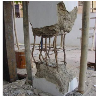
Fig-1.2: Failed Soft Storey Column.
