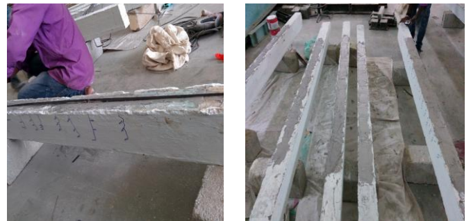
Fig -1: Installation of FRP in groove on tension side and finishing with epoxy adhesive
