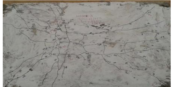
Fig -3.2: Typical crack pattern of SCC slab (tension side)
