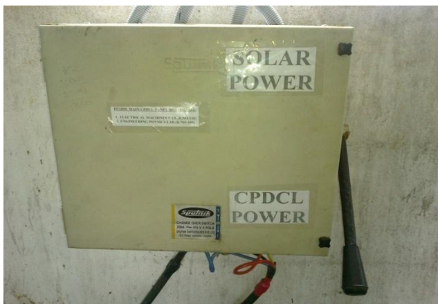
Fig: 14: CPDCL to Solar power exchanger
