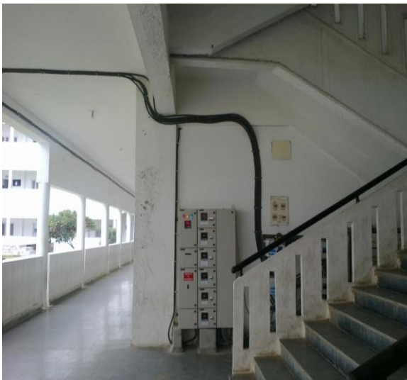
Fig.6: Power cable from PCU to distribution board
