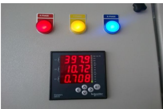
Fig: 8: Solar power Indicator
