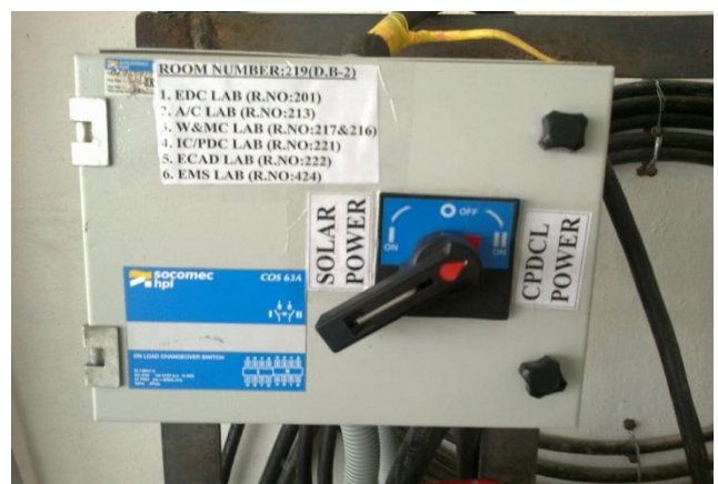
Fig: 11: Solar and CPDCL power distribution
