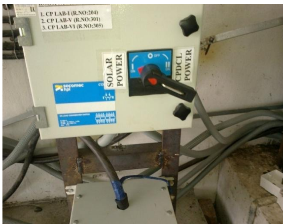
Fig: 13: Solar and CPDCL power distribution
