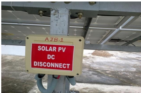
Fig.2.b: Details of Solar panels
