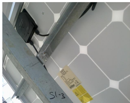
Fig.2.a: Details of Solar panels
