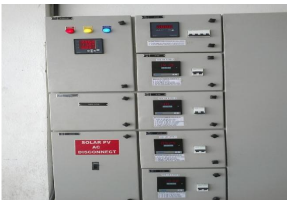
Fig: 7: power Distribution board
