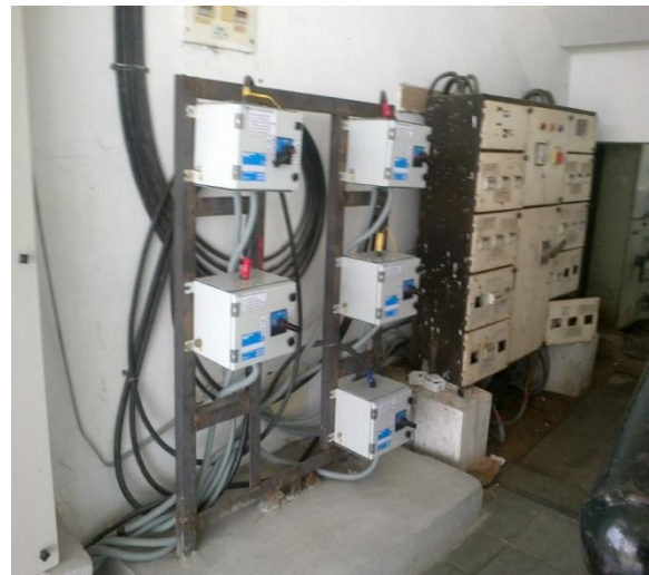
Fig: 9: solar power connected to Distribution boards
