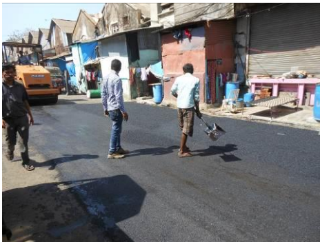
Fig.2: Uneven Paving of Surface coarse by Paver Machine
