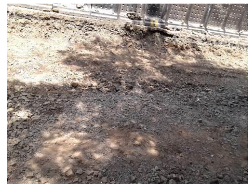
Fig.4: Improper levelling (dressing) at the subgrade layer
