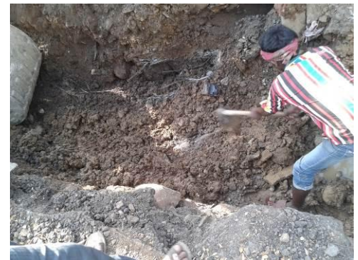
Fig.3: Wirelines/Electricity cables cut off due to improper excavation by Backhoe Loader (JCB)
