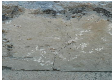
Fig. 8 Failure due to Impact test
