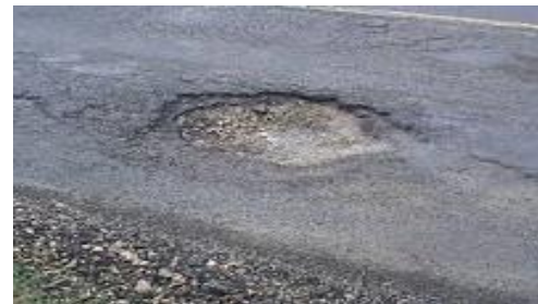
Fig: Selection of potholes
