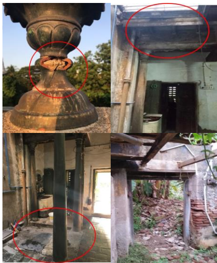
Fig -2: Defects in materials
