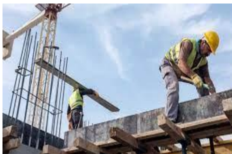
Fig -1: fell down while casting beam
