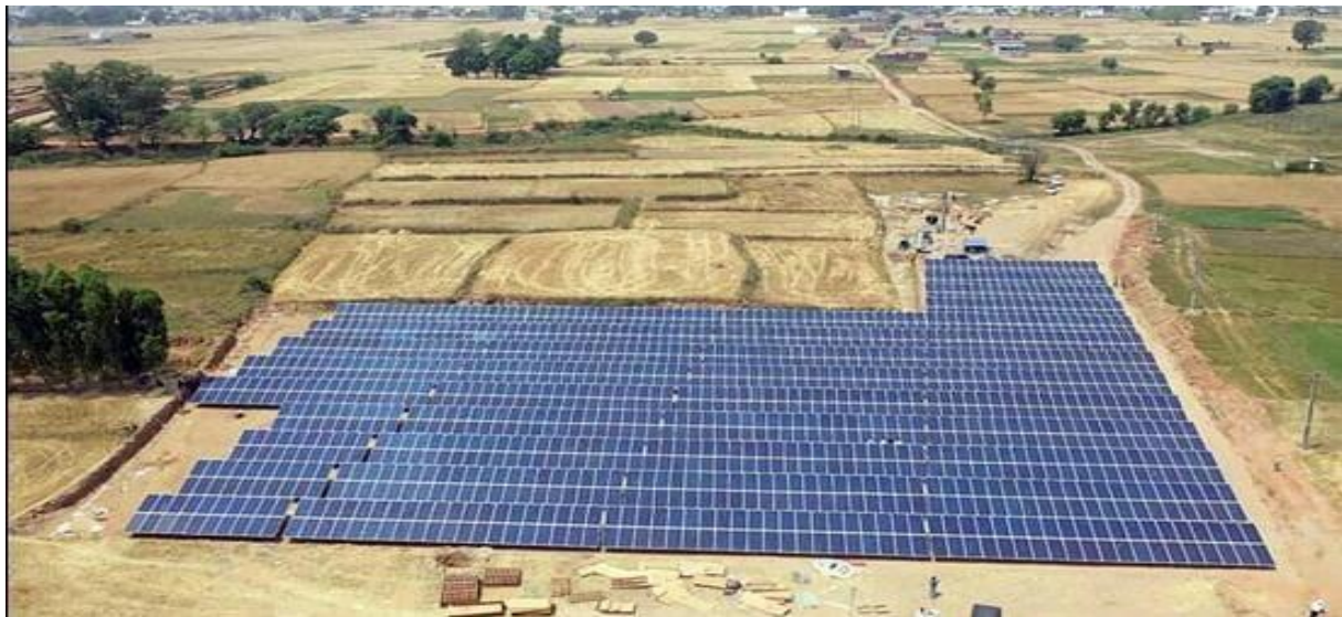
Fig. 1:solar power plant{500 kw}
