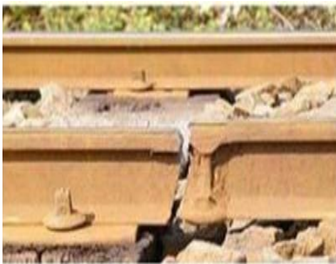
Fig. 1: Crack on track
