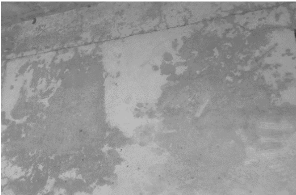
Fig.3.2.2.1 Seepage At Wall Of Building.
