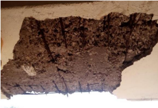
Fig 3.3.1.1 Defects At Building.
