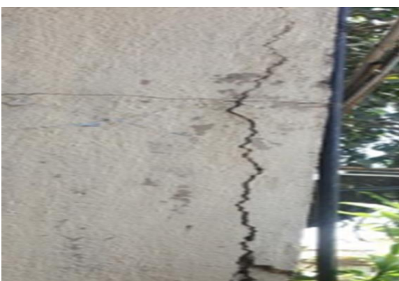
Fig 3.3.3.1 Structural cracks of concrete
