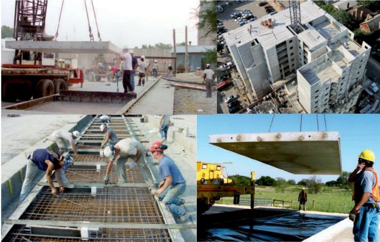
Figure 1: Precast solid slab stripped out of precast bed (top left), precast building erection (top right), tying reinforcement on the form bed in plant (bottom left), erection of slab at job site (bottom right) , Picture from PCI 8 th Edition [2]
