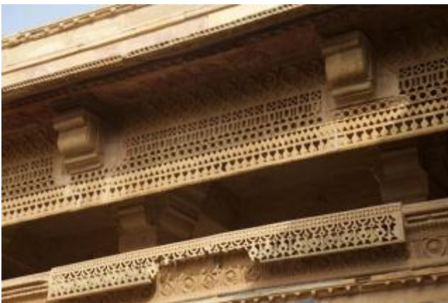
Figure 8 Image showing massive brackets supporting chajja in courtyard of Man Mandir Palace (Source- Google Earth)
