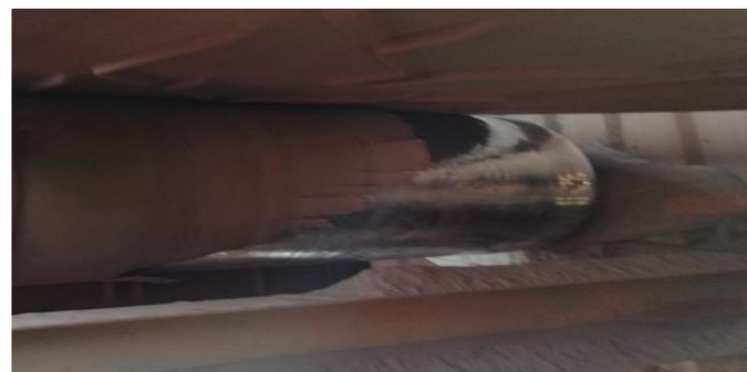
Fig -4: Wear & Tear of Bend Pulley Lagging
