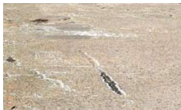
Fig-2: Water & salt crystals in cracks in a car park
