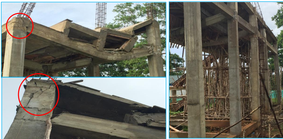
Figure 3. a. Concrete Column Structure the top cracks and crumbles, b. Concrete Column Structure central section and the bottom is still good not to have cracks
