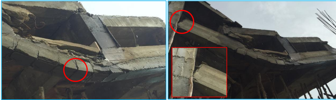
Figure 2. a. 1st floor concrete block concrete blanket does not exist, b. The number of reinforcements of the upper beam pedestal is visible only.
