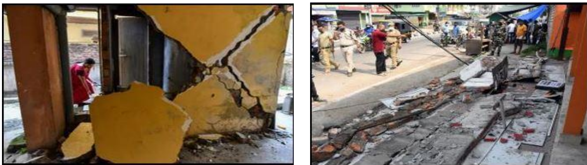
Fig. 2. 28 April 2021 Sonitpur (Assam) Earthquake (Magnitude 6.4), diagonal shear cracking and subsequent collapse of masonry infill wall and out-of-plane collapse of masonry parapet walls.
