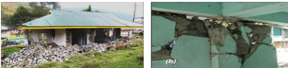
Fig. 3. Sikkim-Nepal Border Earthquake of September 18, 2011 (Magnitude 6.9), (a) Damaged masonry building wall of the police check post at Lachung. (b) Damage to storage facility building wall in Chungthang.
